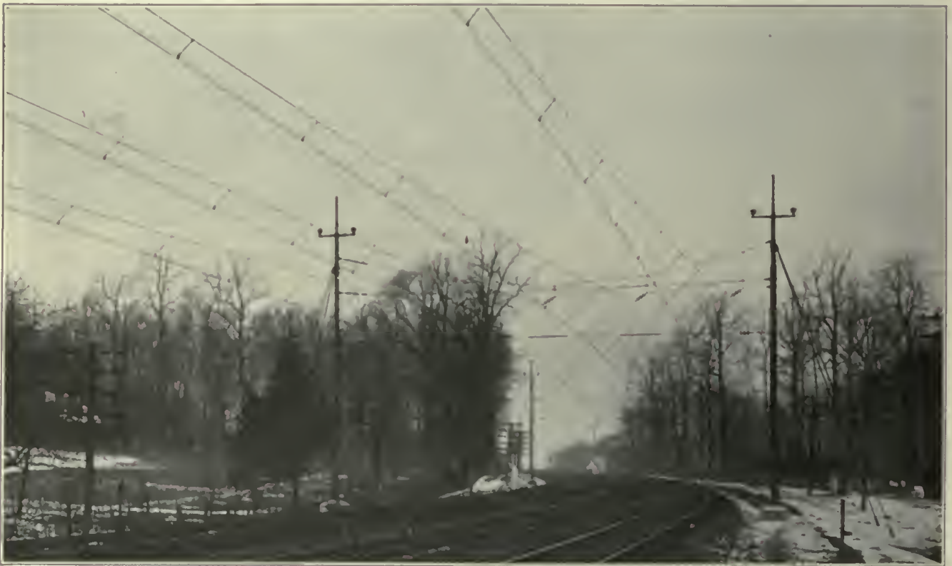
FIG. 514. OVERHEAD CONTACT SYSTEMS. Single Catenary Overhead Contact System on Curve. 11,000-Volt Single-Phase Main Line Construction, Pennsylvania Railroad, near Philadelphia, Pa.
